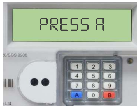
Smart meter screen & keypad
